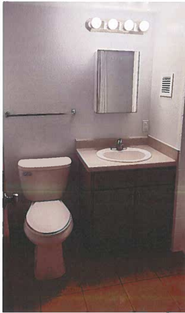
Bathroom vanity, lighting, toilet
